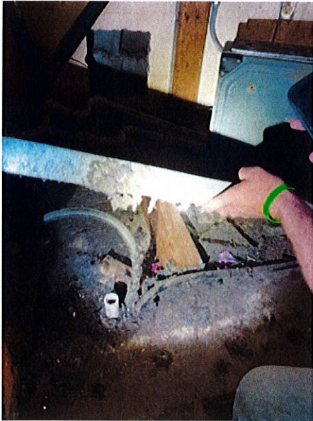
9 - HVAC EQUIPMENT AREA with possible ACM.
