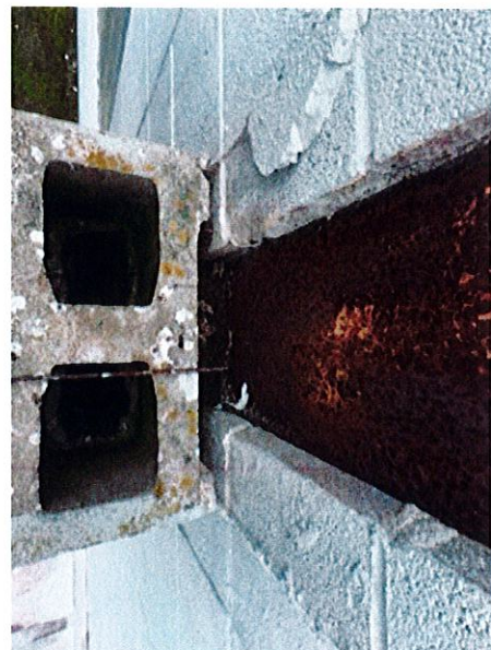
2 - NORTH WALL PILASTER showing lack of filled cells.
