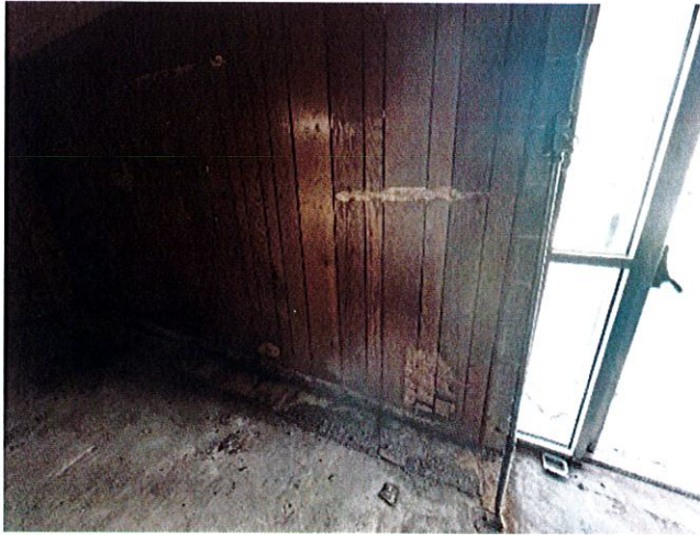
5 - TERMITE DAMAGED AREA near LOBBY.
