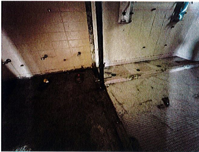
7 - EXPOSED VENT PIPE at LADIES RESTROOM.
