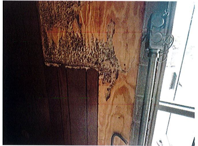
6 - TERMITE DAMAGE behind PANELING.
